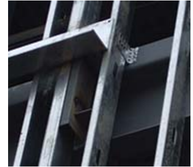
Steel stud cavity and continuous steel brick ledge at floor line where Thermafiber ® Safing Insulation will be installed
